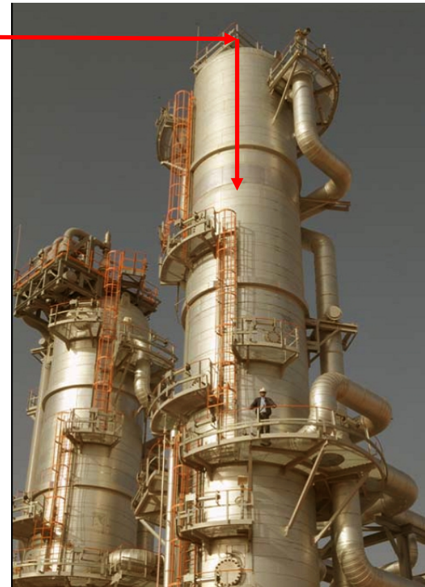
Amine contactor towers
